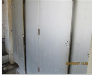
Photo of the sanitary facilities Toilet and hand washing facility (1).JPG
