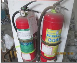
Photo of fire safety equipment Fire extinguishers.JPG
